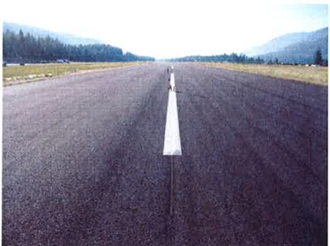
R-11, Surface detail with crack
