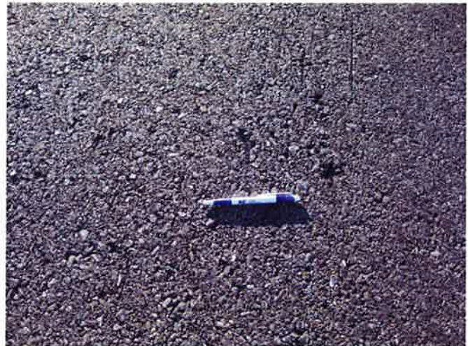
T-11 , Surface detail with raveling
