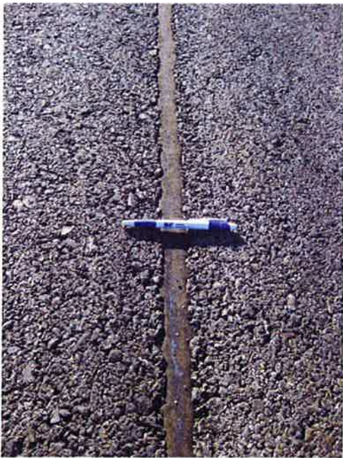
T-11 , Surface detail with crack
