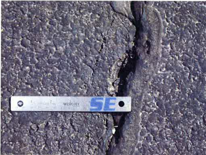
R-1, Surface detail with crack
