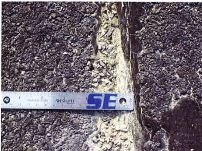
T-1, Surface detail with crack
