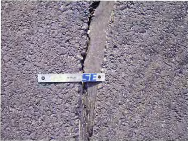
T-3, Surface detail with crack
