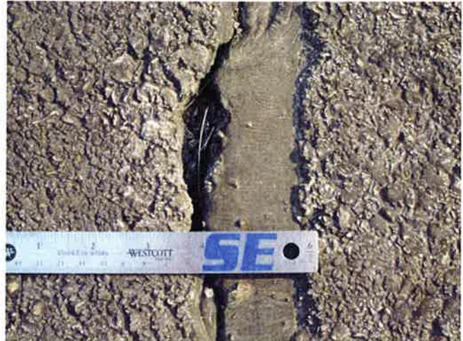
A-1, Surface detail with crack
