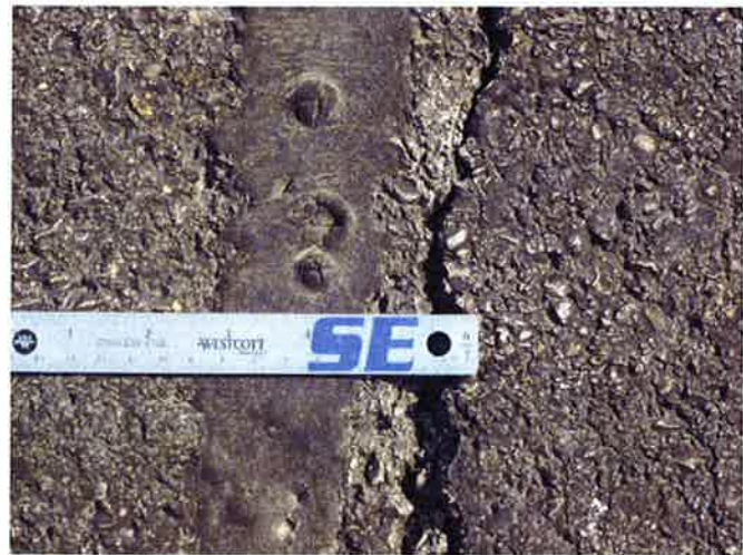
R-1, Surface detail with crack 3
