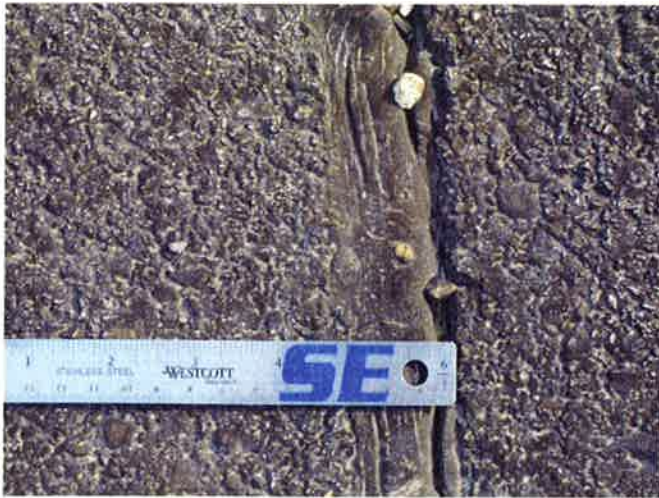
A-2, Surface detail with crack
