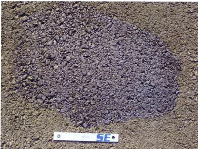
A-1, Surface detail with oil spill
