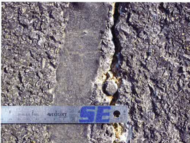
R-1, Surface detail with crack 2
