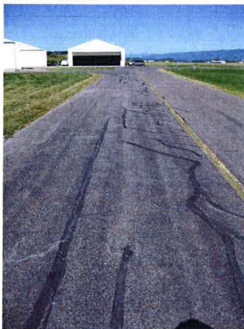
T-12 , Overview with cracks
