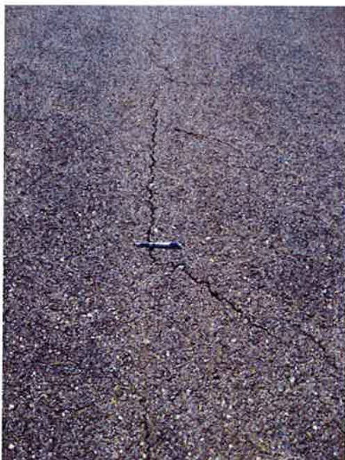
R-11 , Surface detail with cracks
