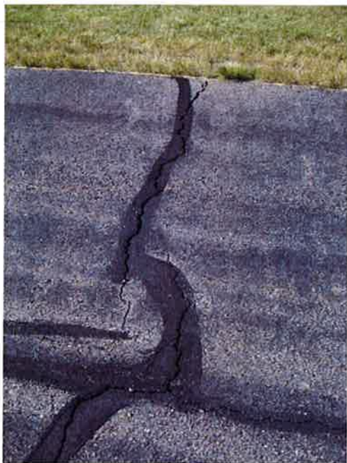
T-11 , Surface detail with cracks
