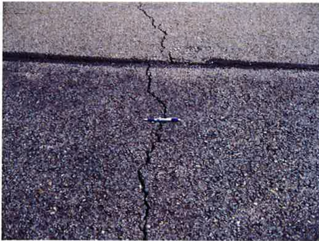
A-11 , Surface detail with cracks
