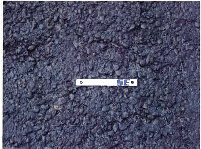
T-1, Surface detail with raveling
