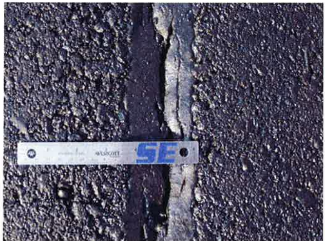
R-4, Surface detail with cracking 2
