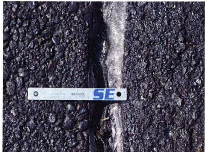
A-3, Surface detail with crack
