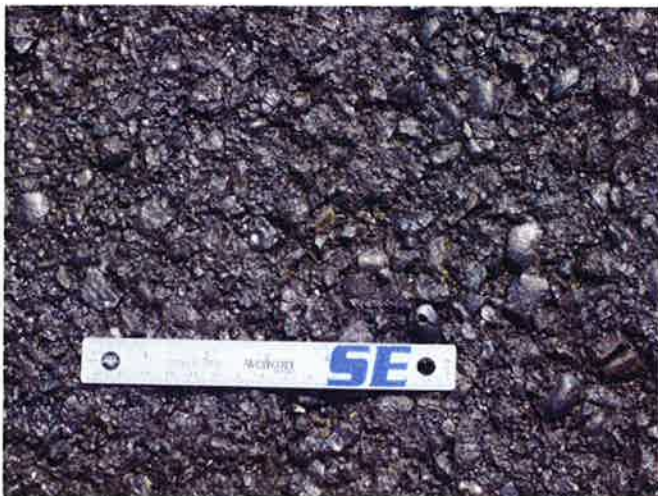
A-3, Surface detail with raveling
