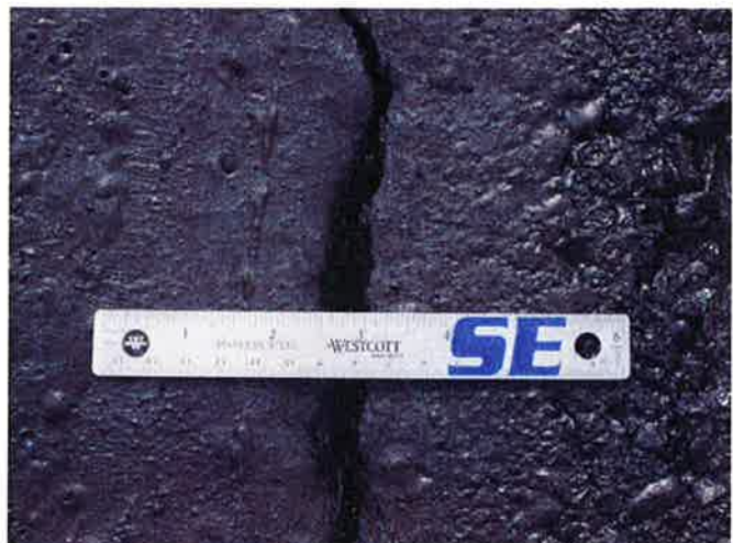
T-1, Surface detail with crack
