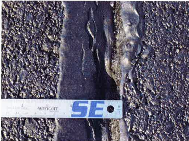
R-4, Surface detail with crack
