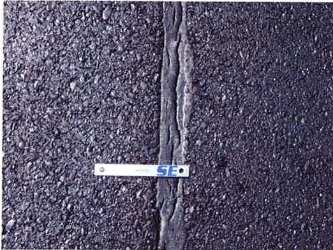
T-9, Surface detail with crack
