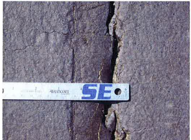
T-8, Surface detail with crack
