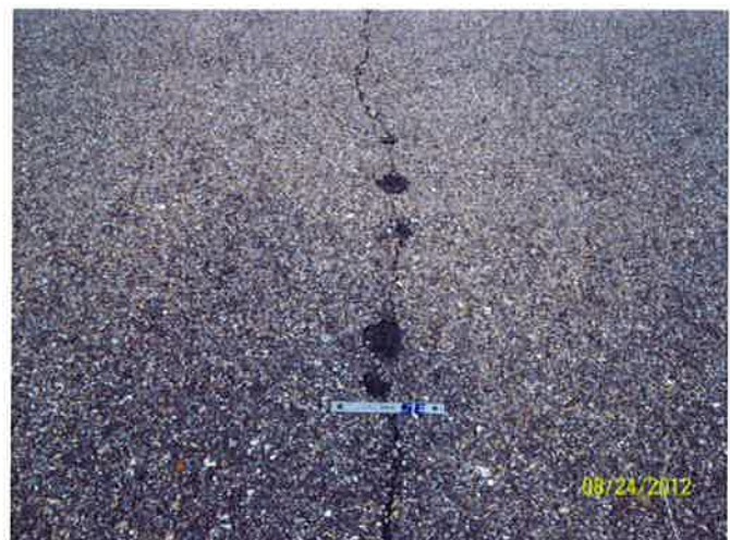
T-1 , Surface detail with cracking and bleeding
