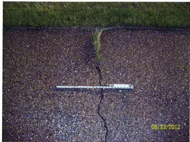
T-2, Surface detail with cracking
