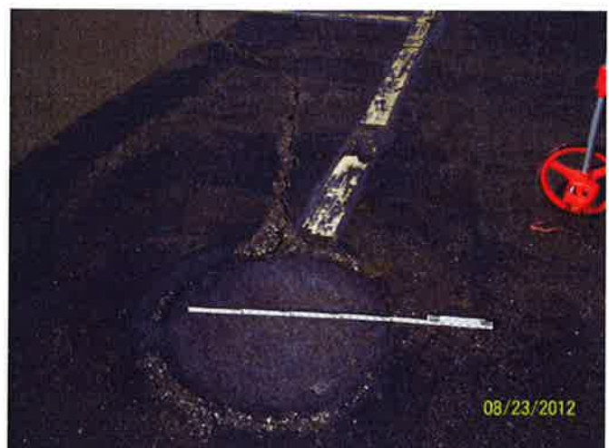
A-2, Surface detail with cracking and patching
