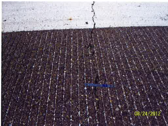
R-2, Surface detail with cracking
