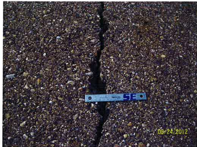
R-3 , Surface detail with cracking
