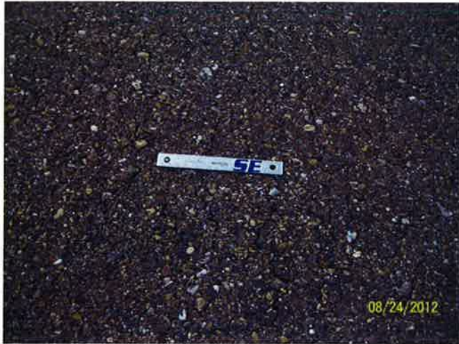
R-3 , Surface detail alligator cracking from over rolling
