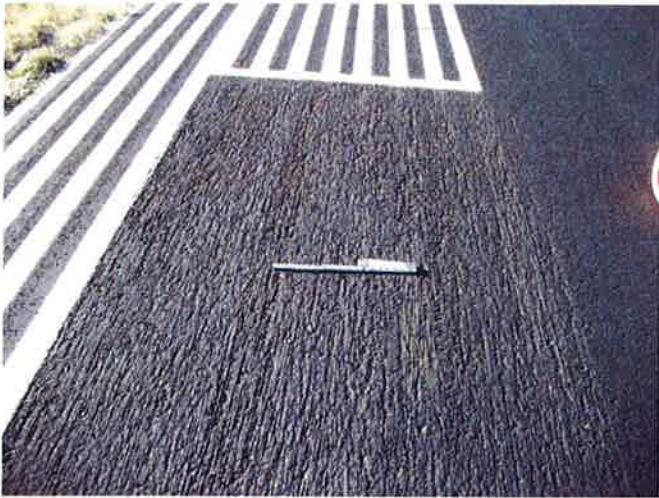
R-21, Surface detail raveling from grinding
