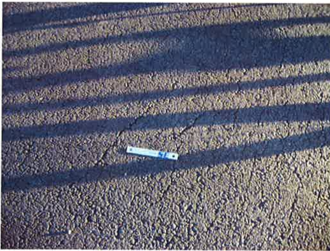
T-5, Surface detail alligator cracking from over rolling
