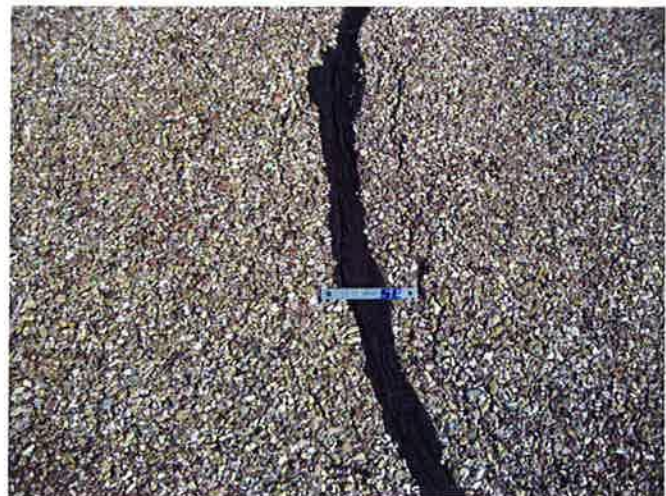
T-2, Surface detail with alligator cracking along transverse crack
