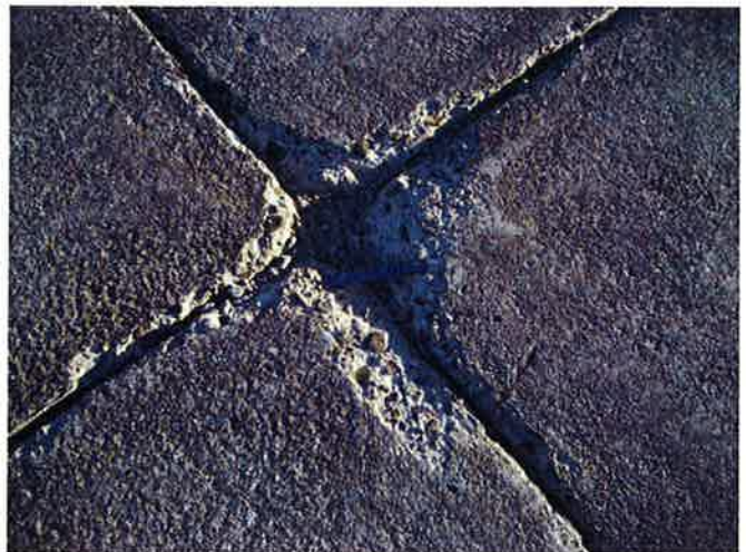
A-1, Surface detail spalling corners
