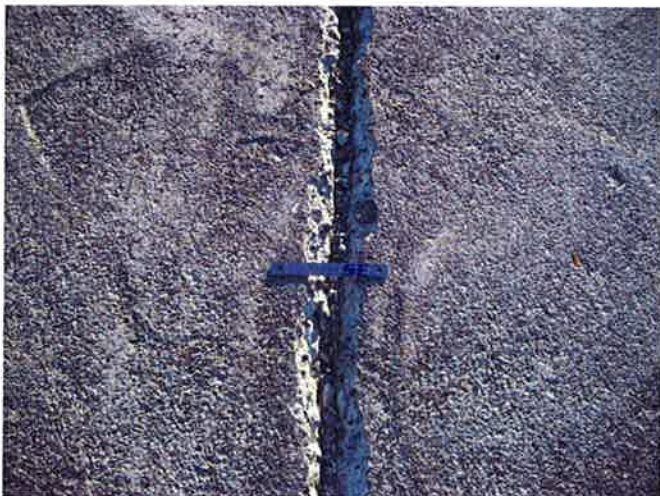
A-1, Surface detail spalling joints
