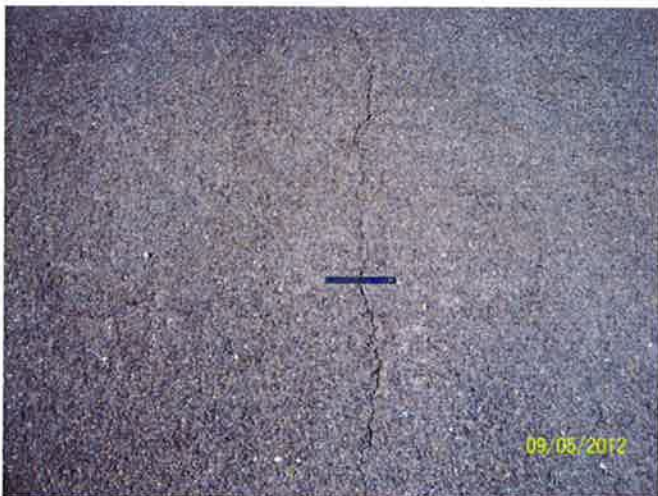
A-1 , Surface detail with crack
