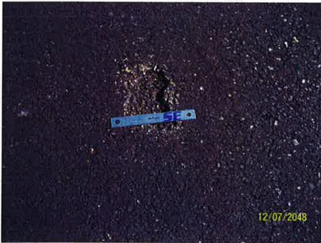
R-1, Surface detail high intensity raveling
