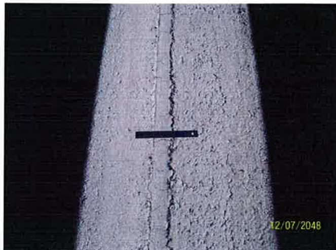
R-1, Surface detail filled crack
