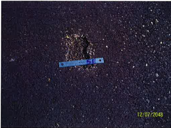
R-1 , Surface detail high intensity raveling
