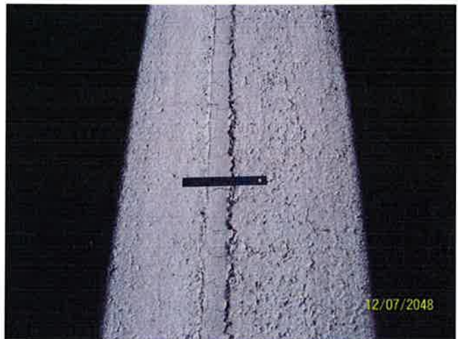
R-1, Surface detail filled crack
